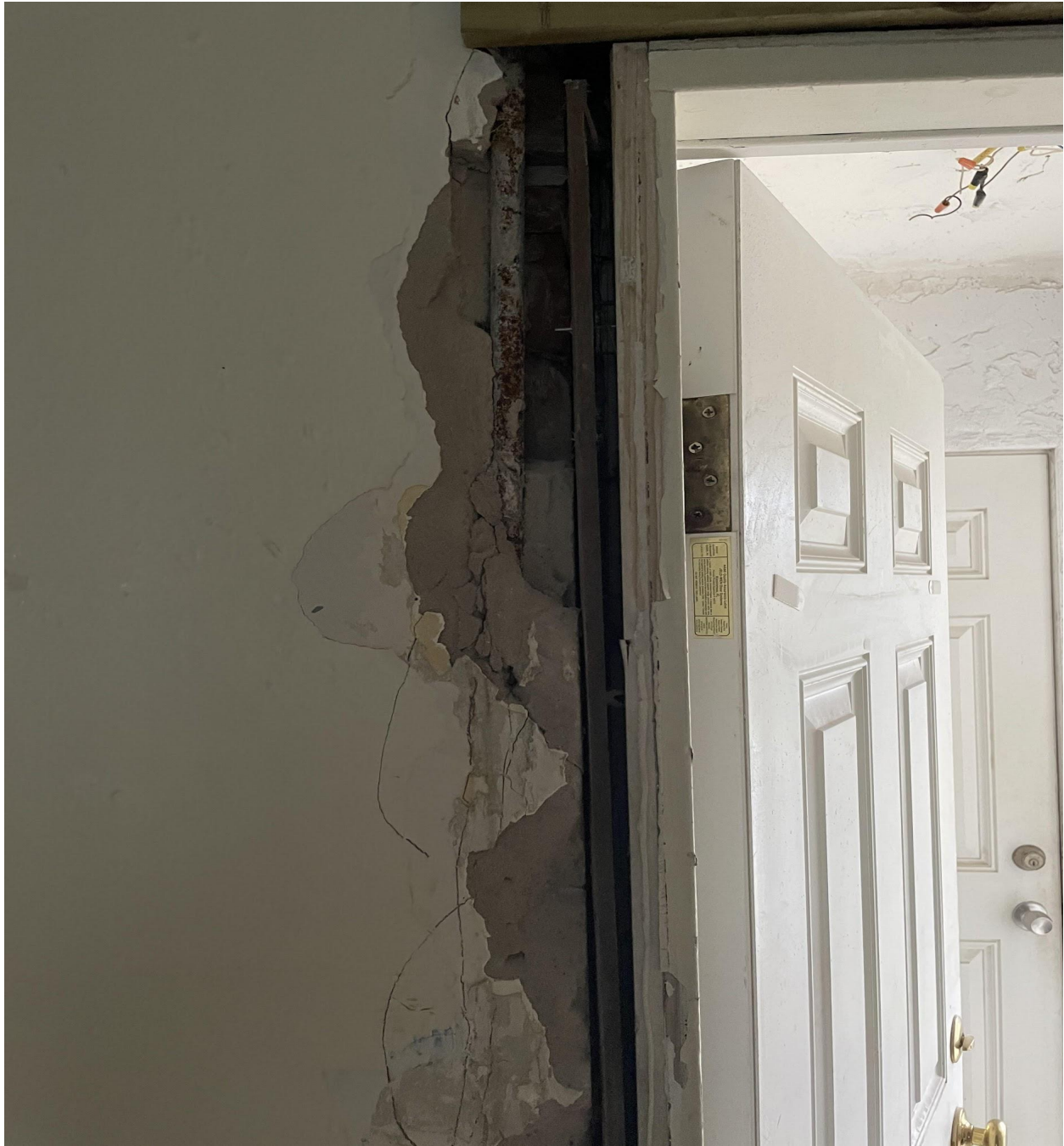
Broken masonry preventing door from being mounted correctly - now repaired
