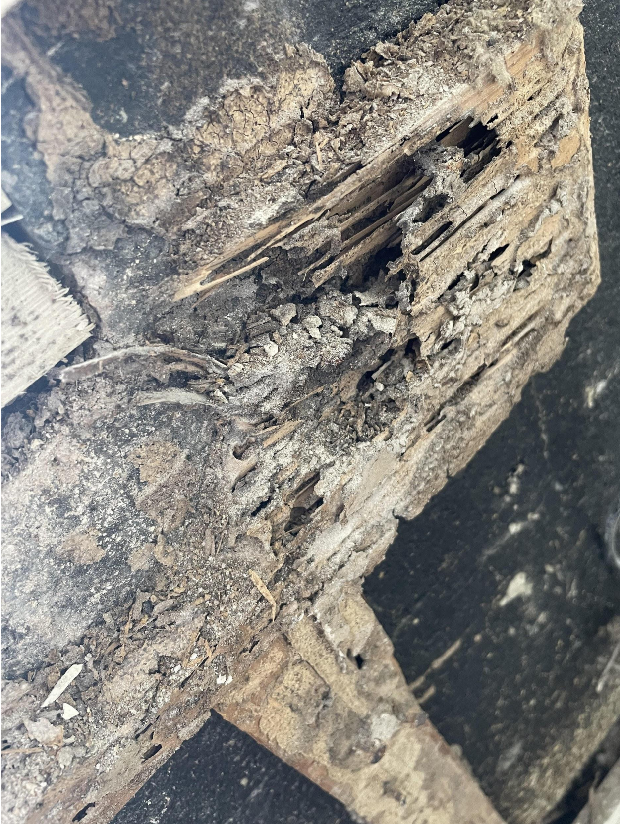
Rot / Mold / termite damage: Example of window leaking down wall from blocked drain
