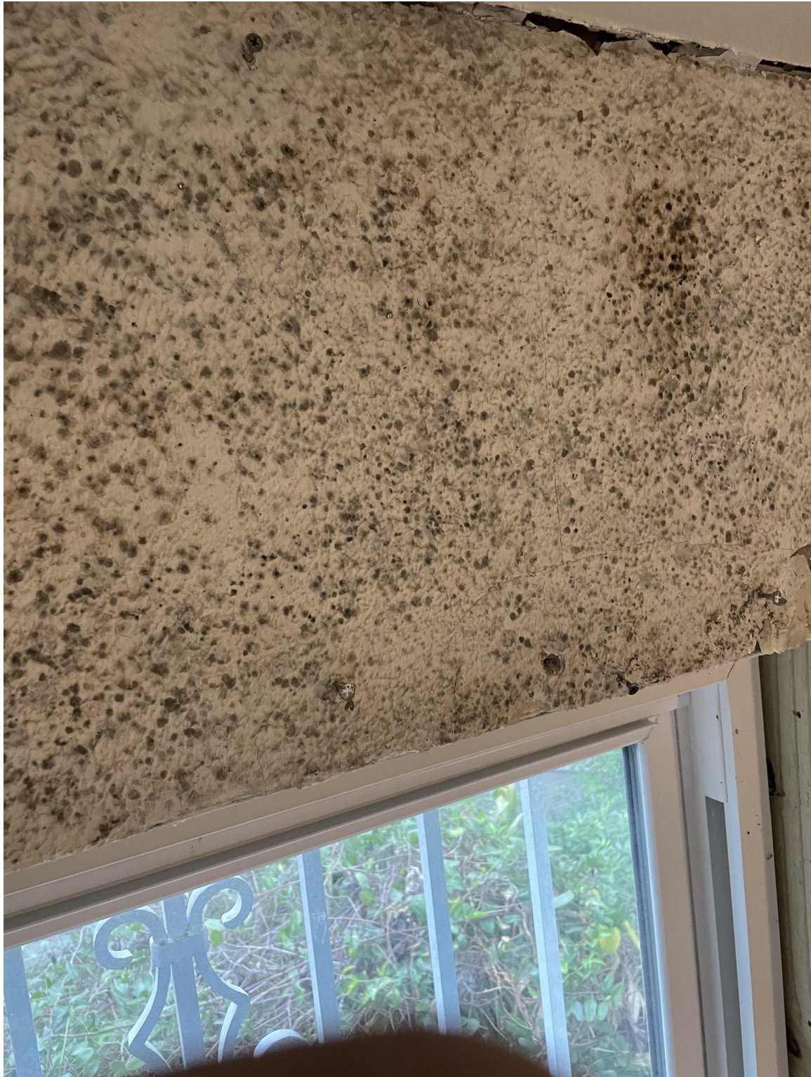
Mold caused by incorrect construction method creating double vapor barrier any walls like this were completely removed and rebuilt.
