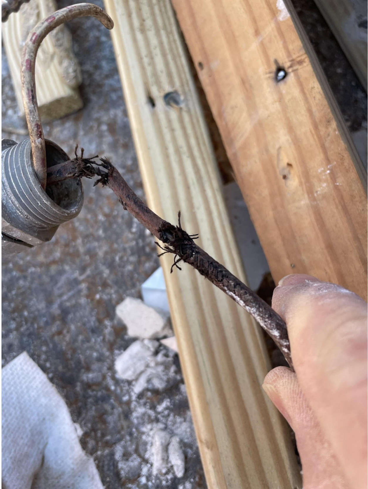
Overheated / burned main feed - rewired - separate circuits feeding individual rms
