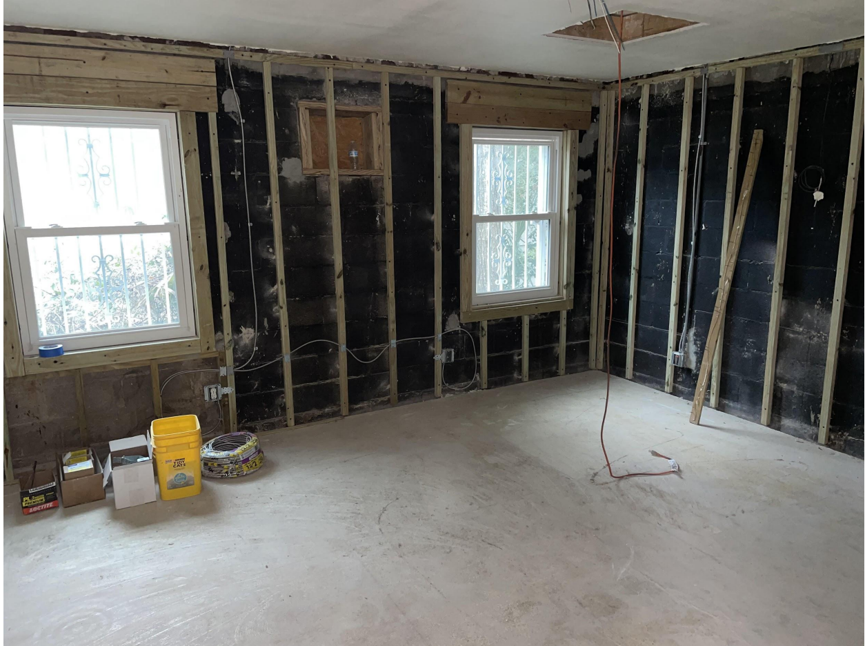
Room 5 refurred/ fire blocked / rewired with added nailer for curtain rod above each window
