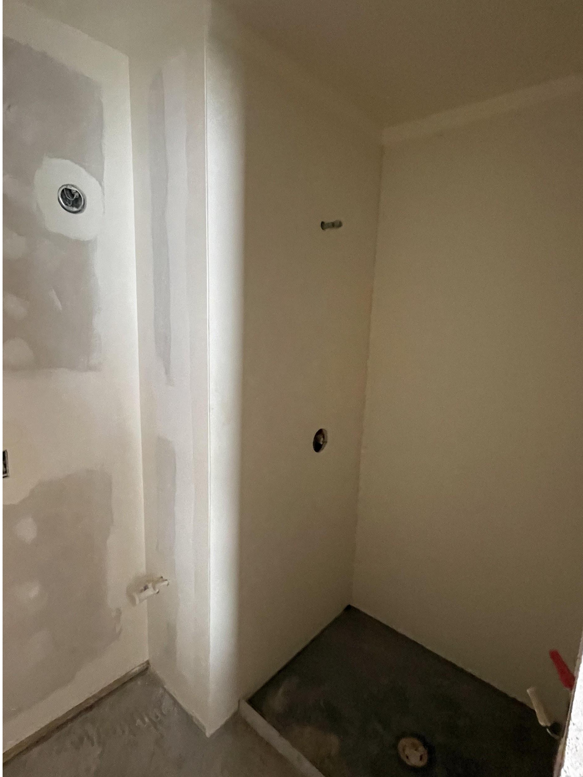
Room 12 bathroom is now painted but showing the picture unpainted shows the shower area better.
