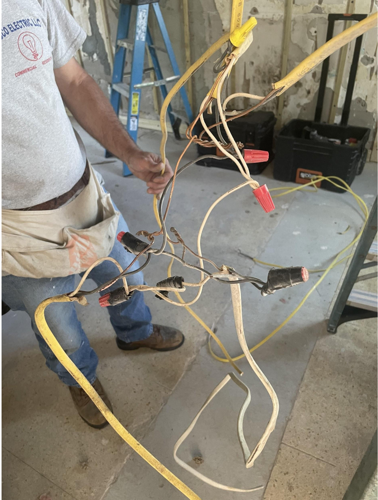
Wires found in attic under insulation
