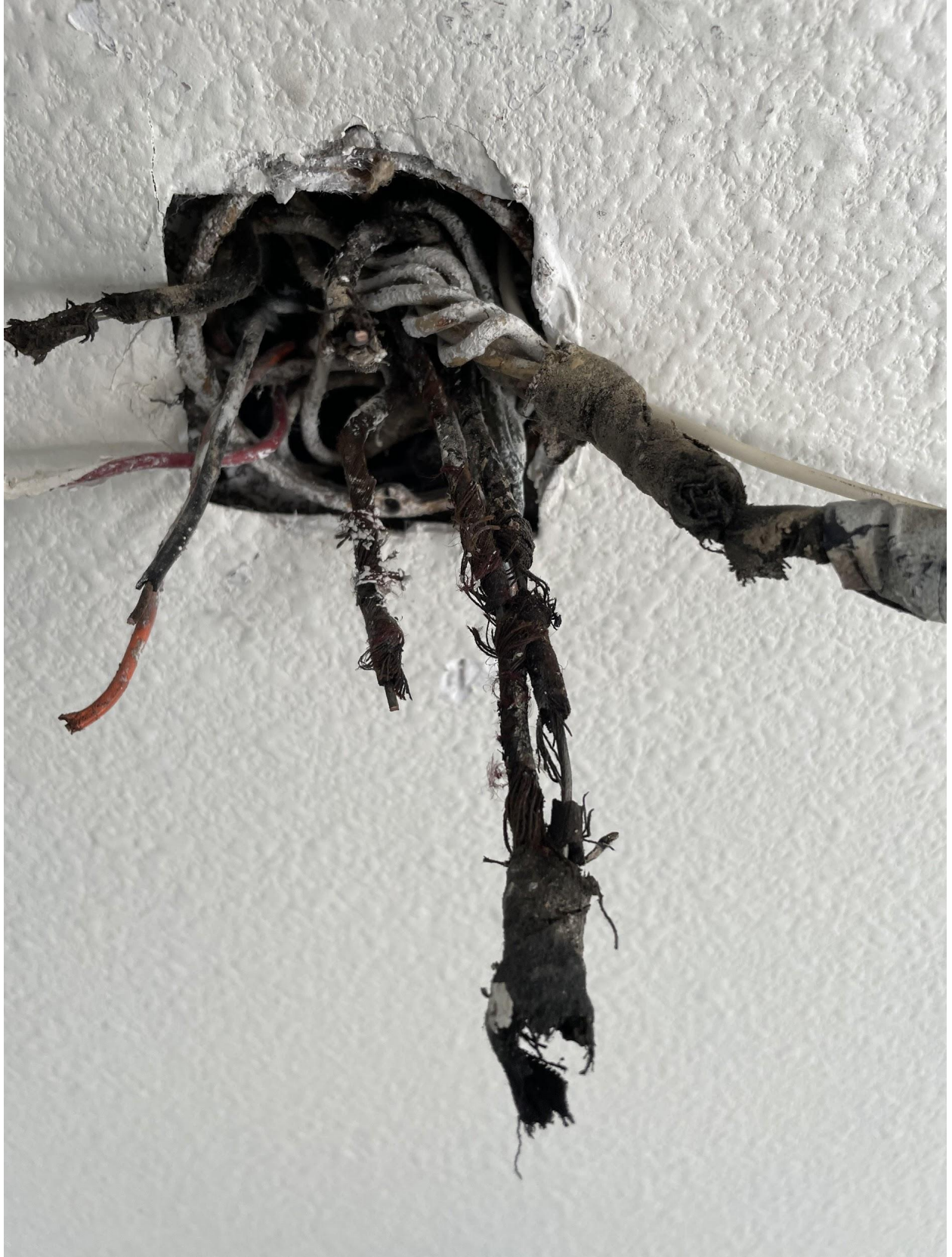
Overloaded electrical fan box with close wire - Note: the broken wire
