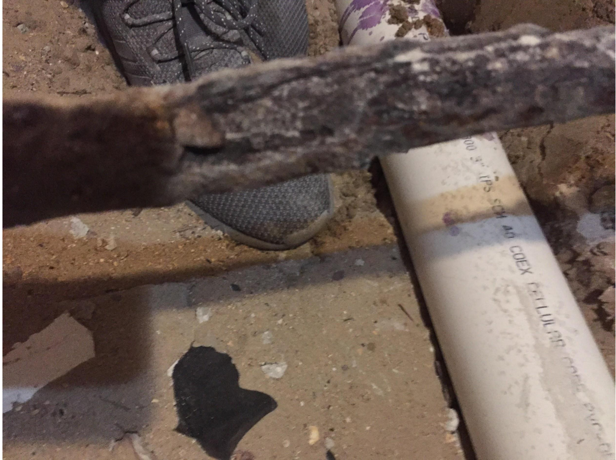
Deteriorated pipe below room 5 slab
