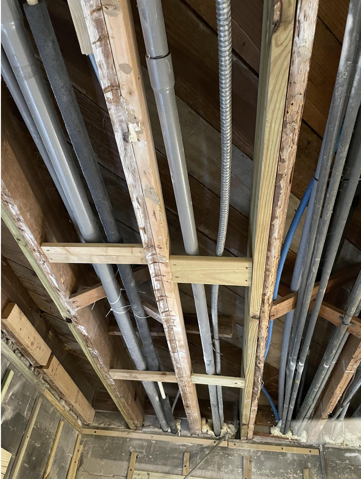
2x10's sistered to termite eaten wood with new electrical conduit added
