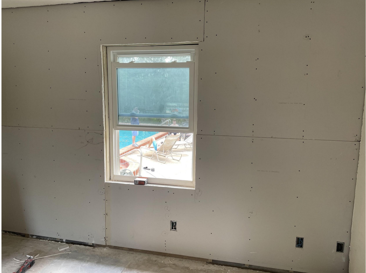
Room 7 back in sheetrock, note added outlet, cat6 wire placement and cable
