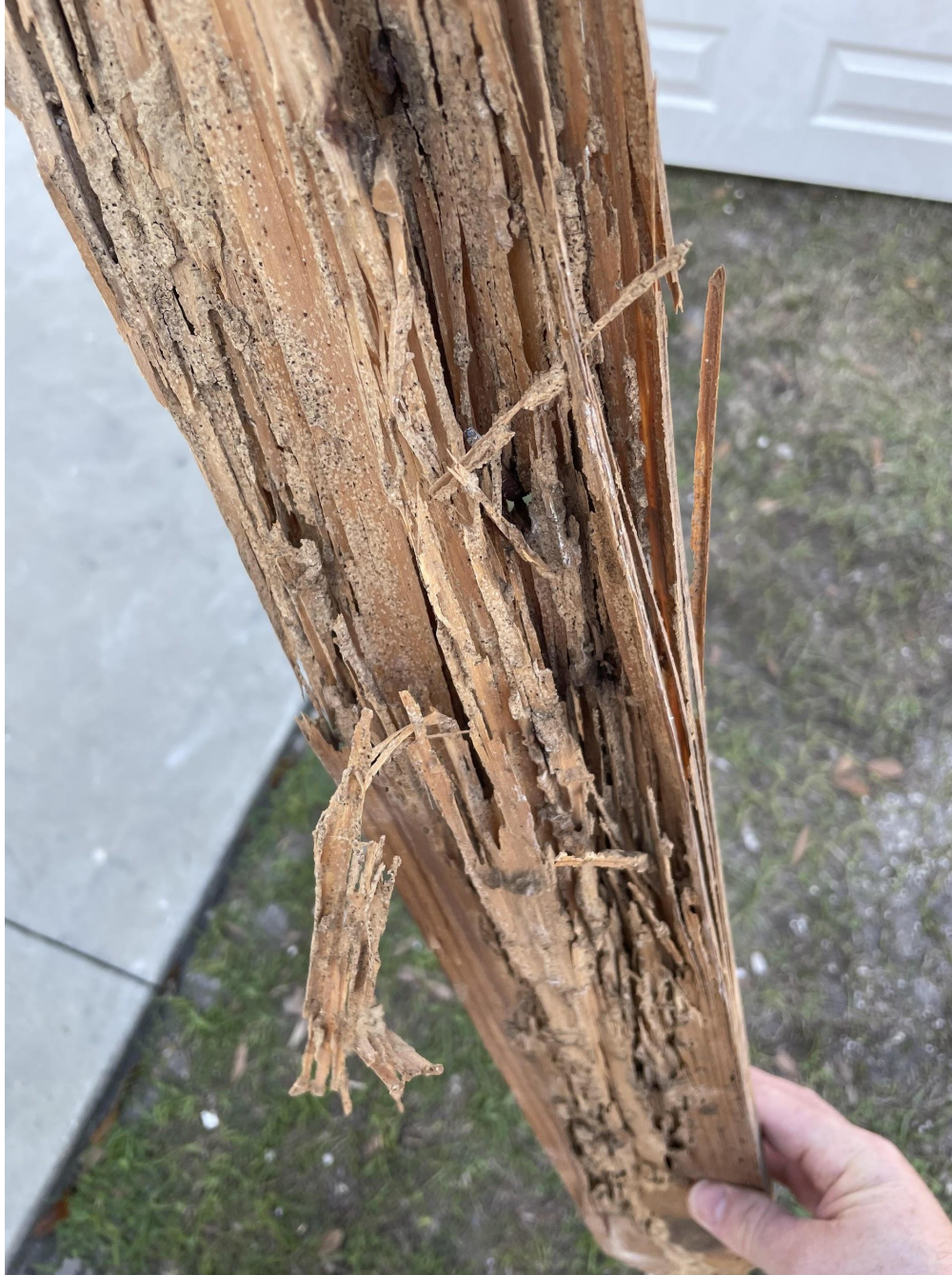
Typical termite damage because the house was not protected properly from insects.
